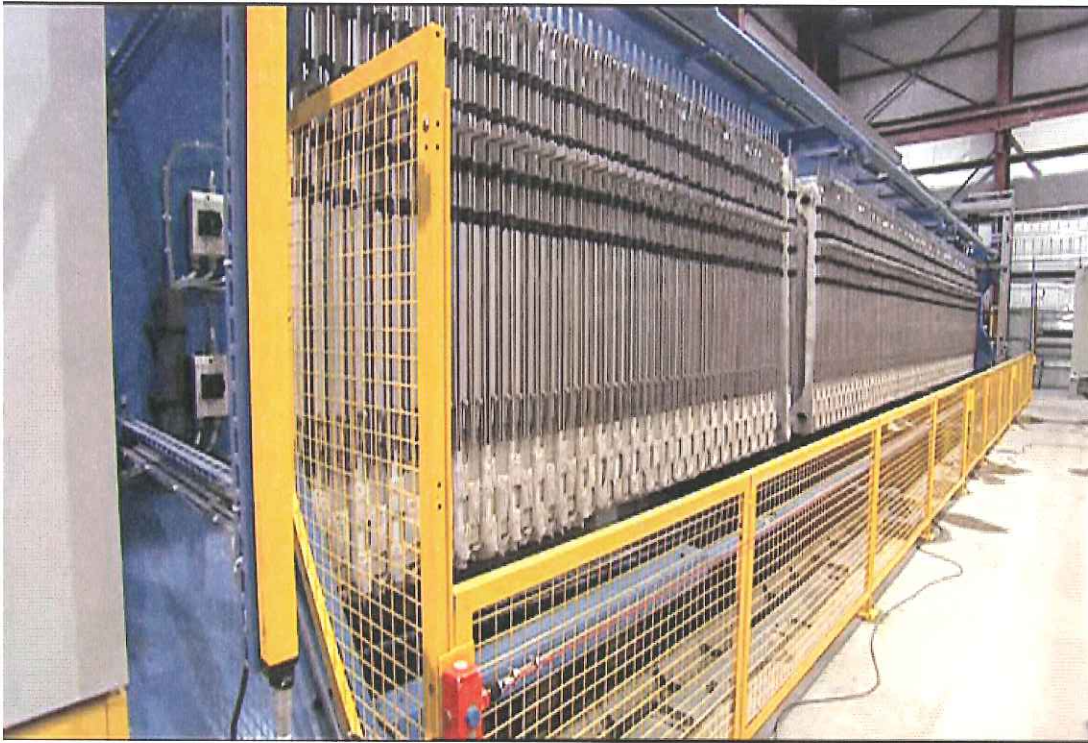
Figure 3. Plate and frame presses for dewatering sediments from OU 2 – 5.
