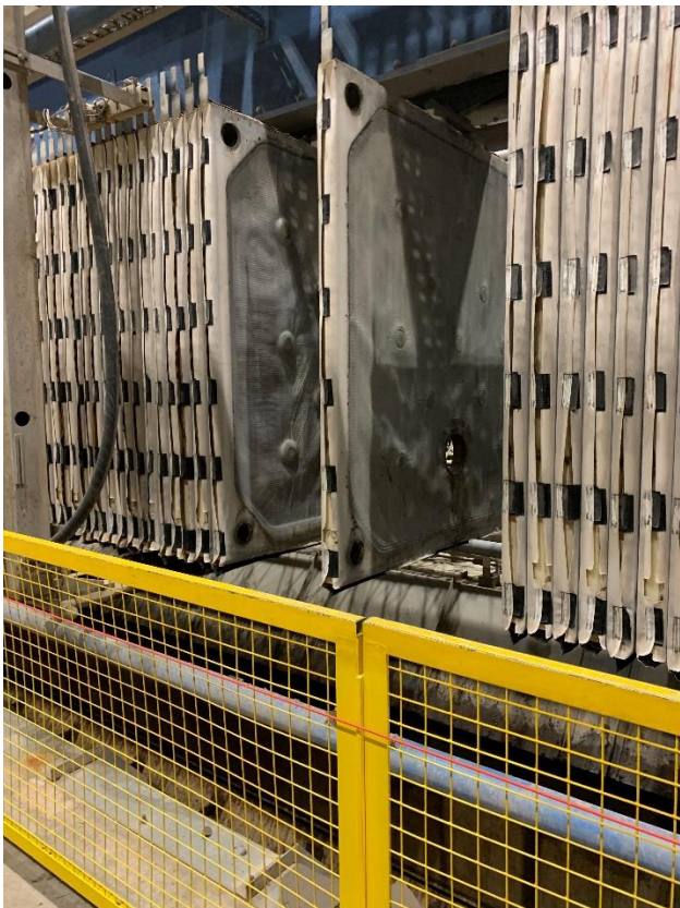
Filter Press in Operation Sediment Dewatering Plant
