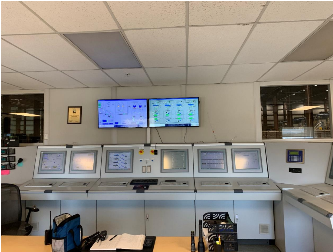
PLC System Sediment Dewatering Plant
