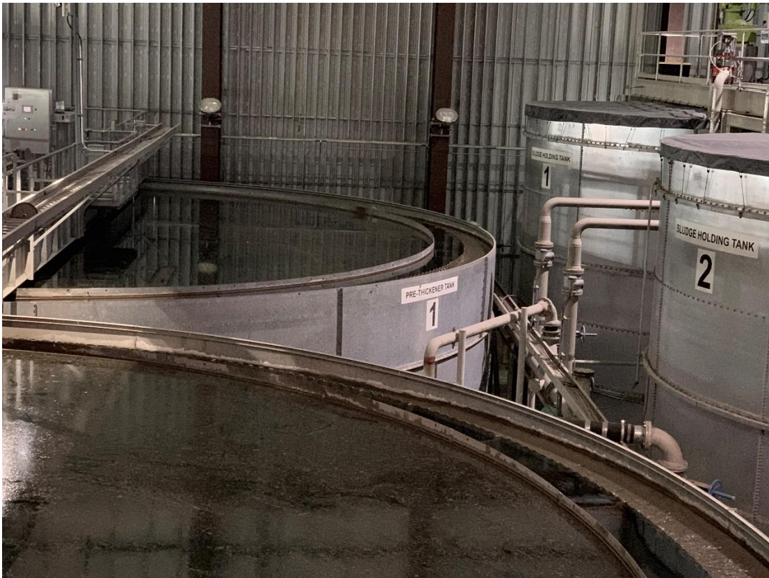
Sludge Pre-Thickener and Sludge Holding Tanks
