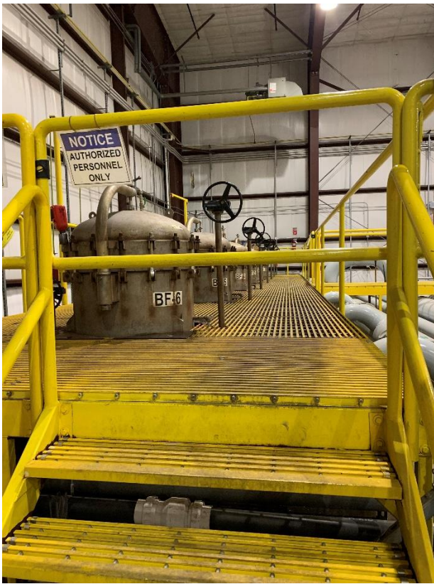
Bag Filters Waste Water Treatment Plant
