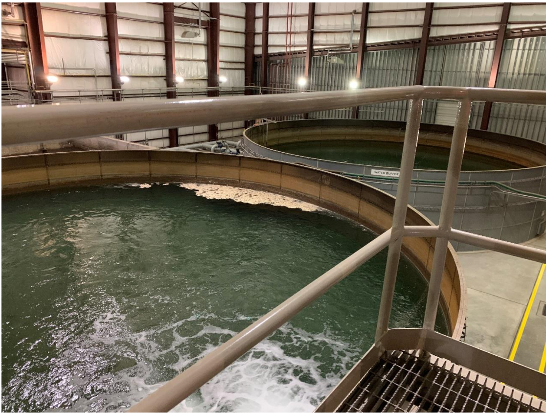
Sediment Dewatering Plant Water Buffer Tanks (clarifiers)
