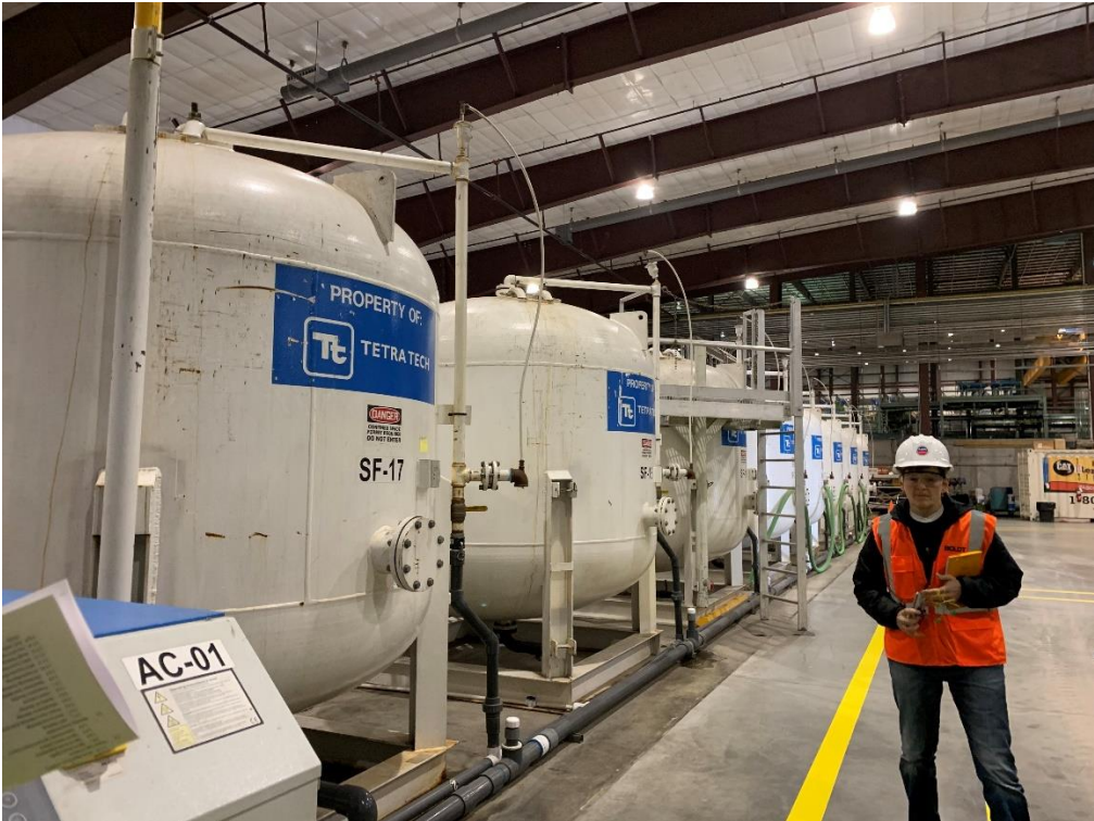
Sand Filters Waste Water Treatment Plant
