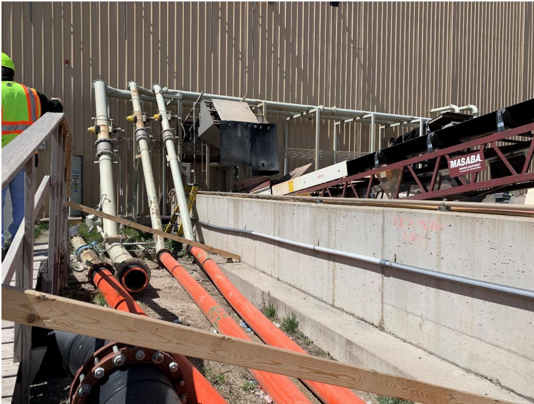
Influent Sediment Sludge (orange lines) and treated water effluent (black line)
