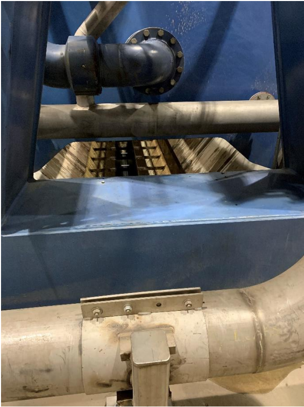
Filter Press Conveyor Belt Sediment Dewatering Plant
