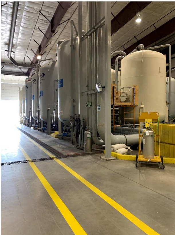
Granular Activated Carbon Polishing Step Waste Water Treatment Plant
