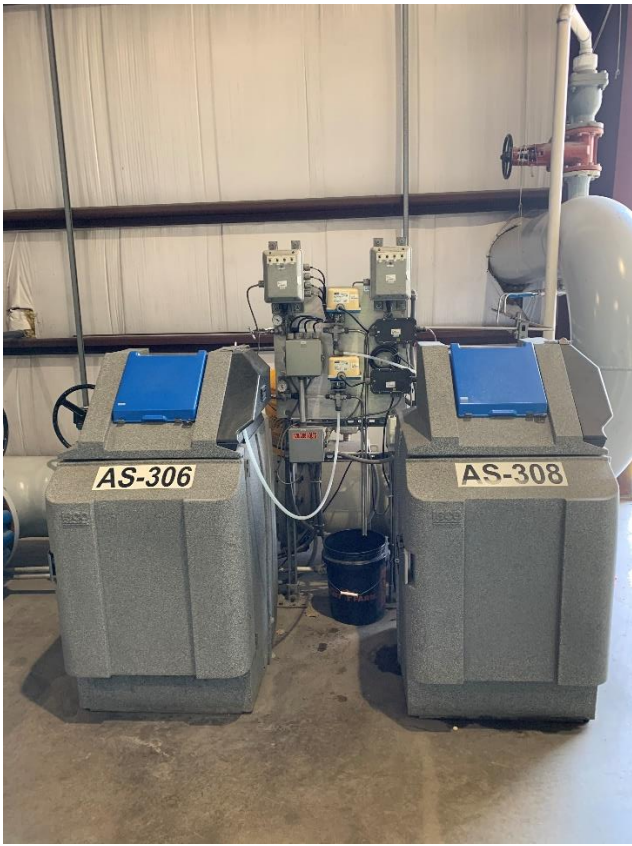
Automatic Effluent Sampler Waste Water Treatment Plant
