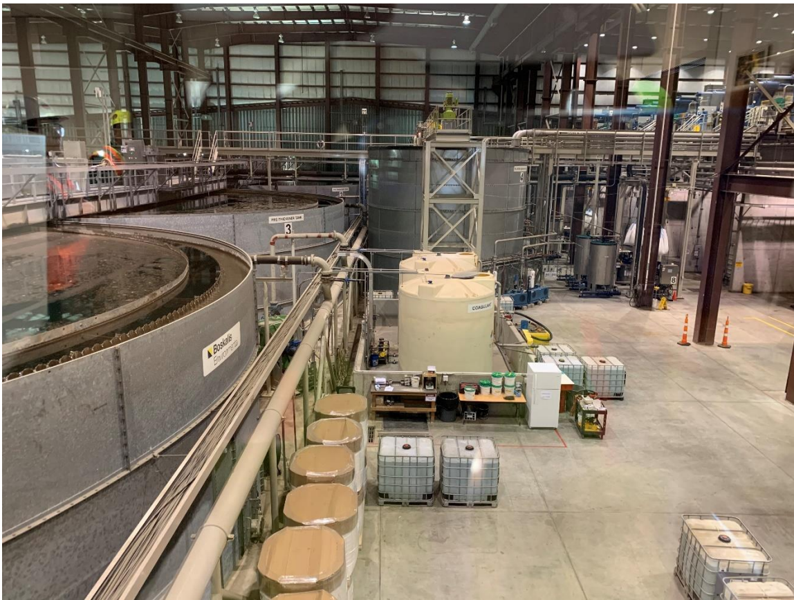
Sediment Dewatering Plant View
