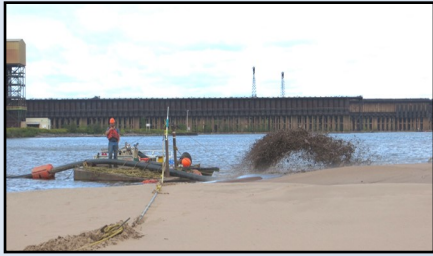
A slurry of sediment/sand mixed with water, and placed hydraulically, created the beach
